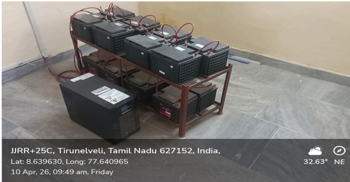
Uninterrupted Power Supply
