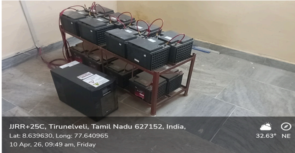
Uninterrupted Power Supply
