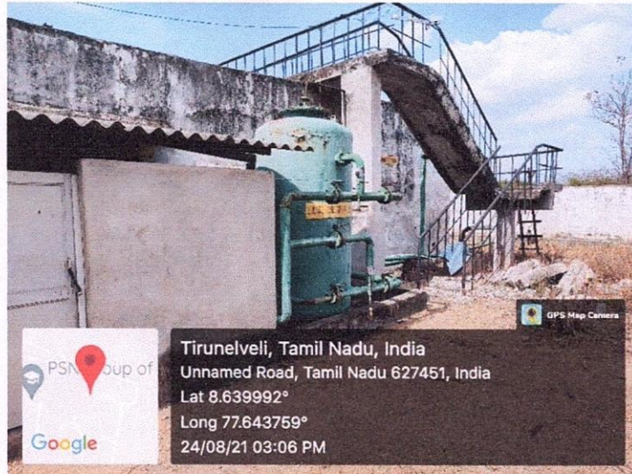
STP Plant at PSNCET Campus
