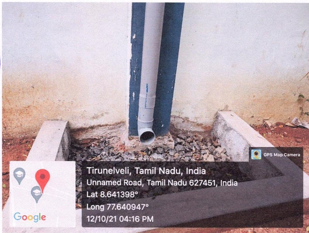
Rain water harvesting Pit in the First Year Block
