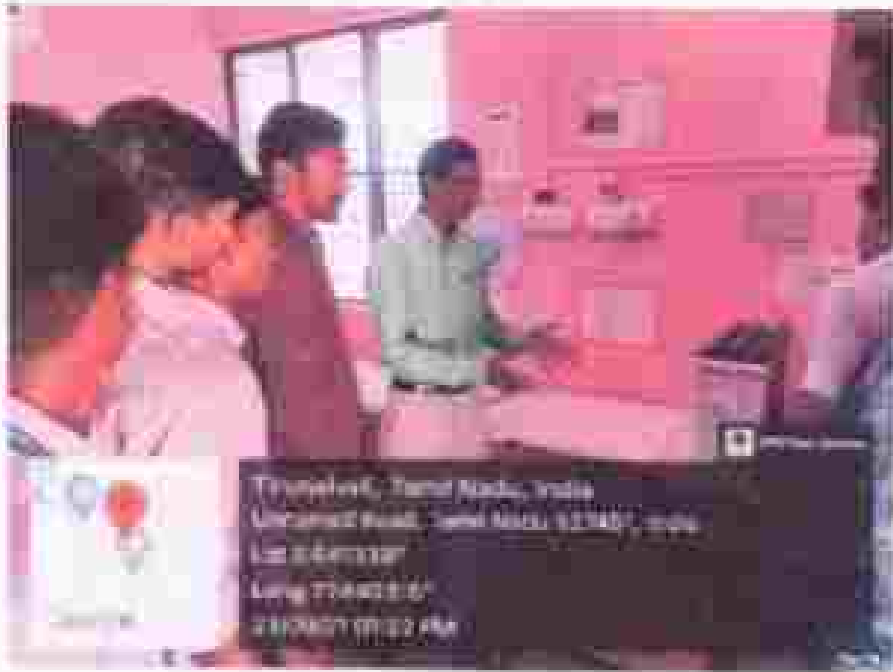
A practical session with students to explain the working of solar PV system
