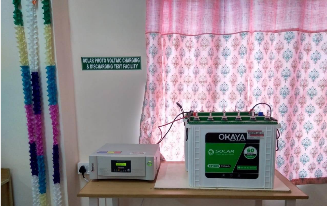
Solar Plant control unit
