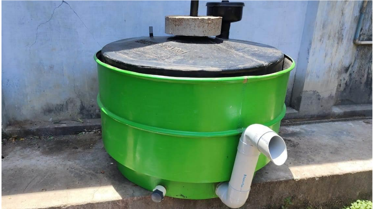
1 M 3 Capacity Bio Gas Plant Installed inside the Campus
