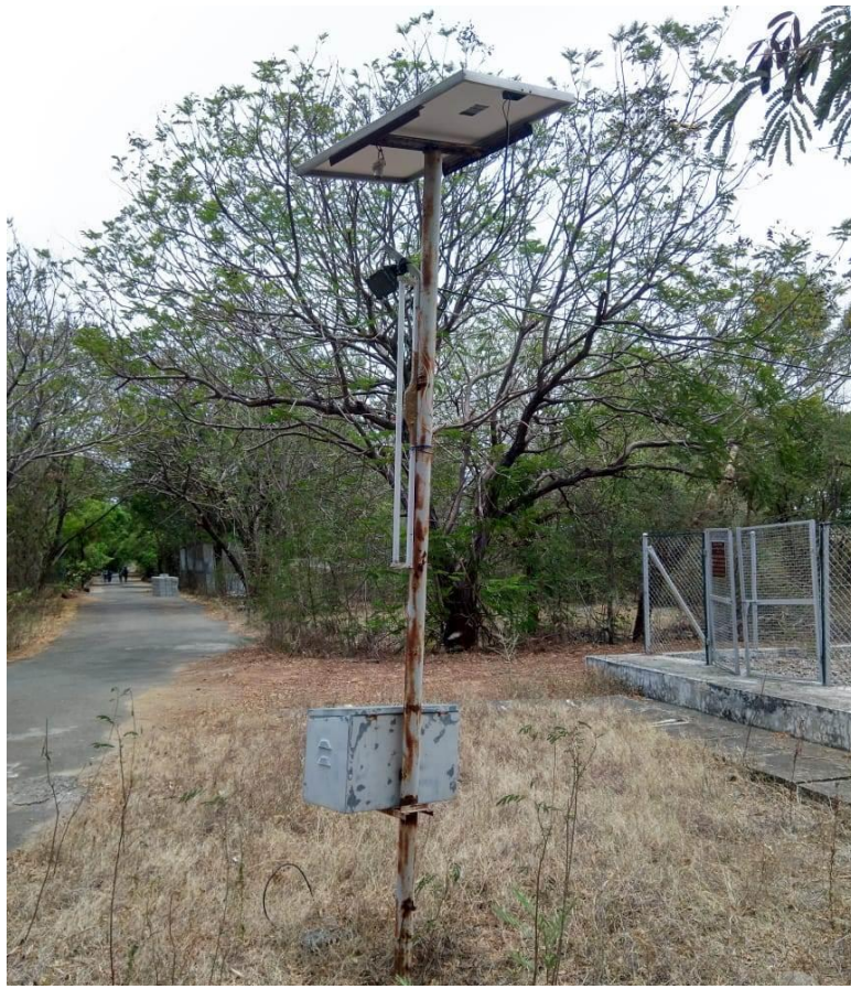
Solar based Street Light are Installed in the Campus
