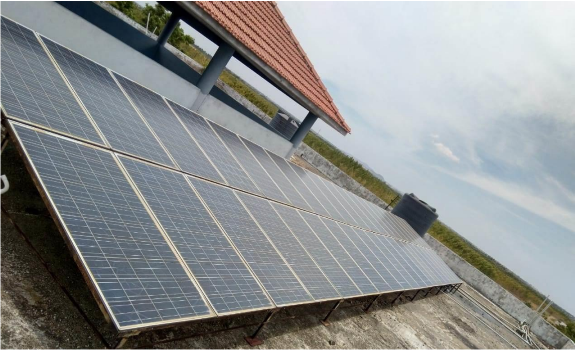
Solar Plant Installed in Roof Top of College Campus
