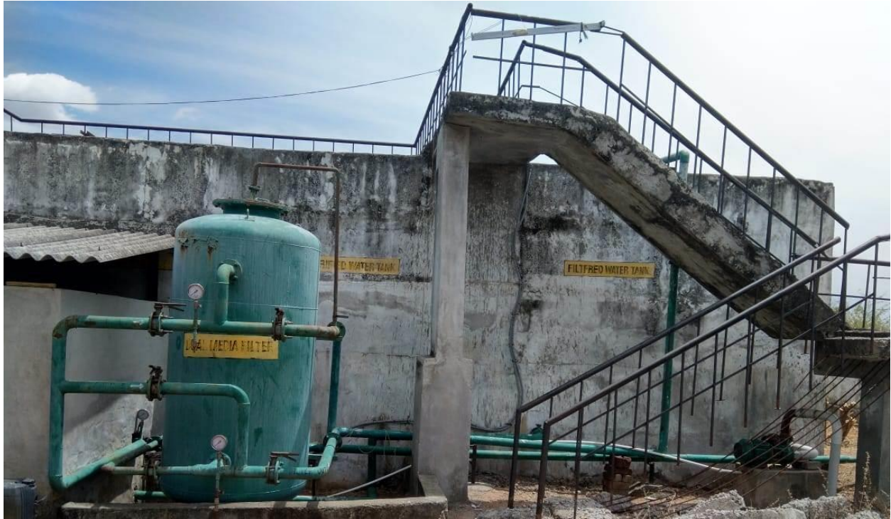
Sewage Treatment Plant Installed in the Campus
