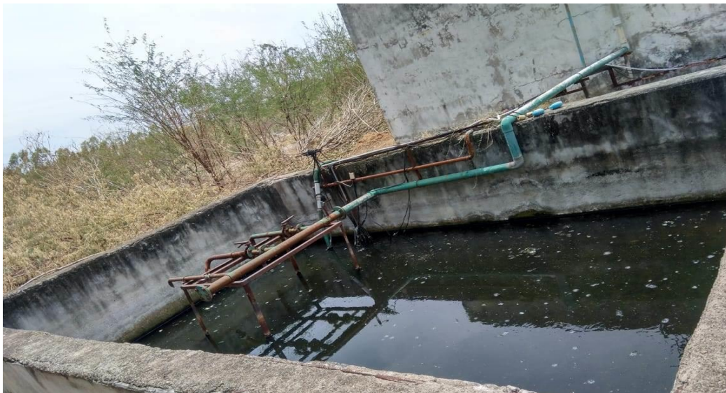
Sewage Settlement Tank
