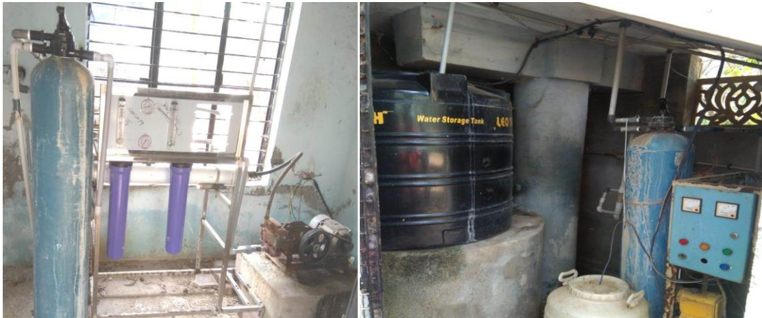
RO Water plant in the Campus
