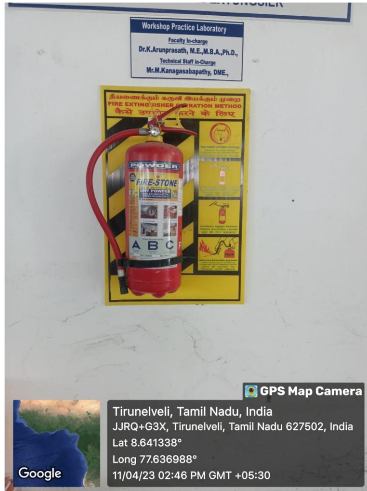
A view of Fire Extinguisher in Academic block
